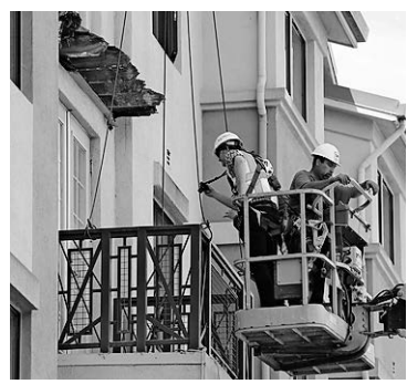
Workers prepare to remove the balcony below the one that collapsed, leaving 6 dead and several critically injured, at the Library Gardens Apartments in downtown Berkeley, June 17, 2015.
